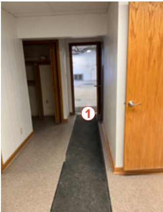
① Floor in historic building will require leveling to meet ADA requirements
