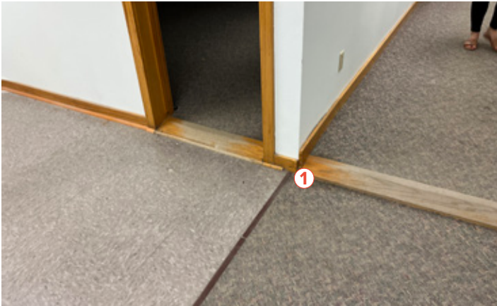
① Floor in historic building will require leveling to meet ADA requirements
